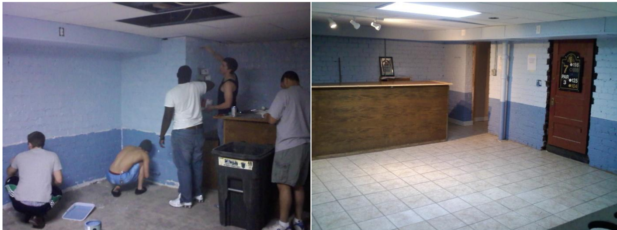
Brothers of Eta Chapter painting the bar room after renovations to tile floor, ceiling, and bar.
