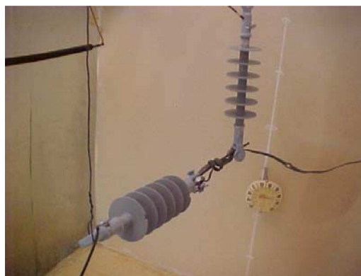
Fig. 1. The 28-kV vertical and horizontal distribution/dead end insulators.
